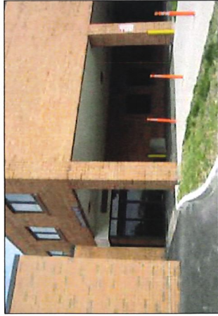
LOCATION: 22 - LACK OF PROPER SIGNAGE
